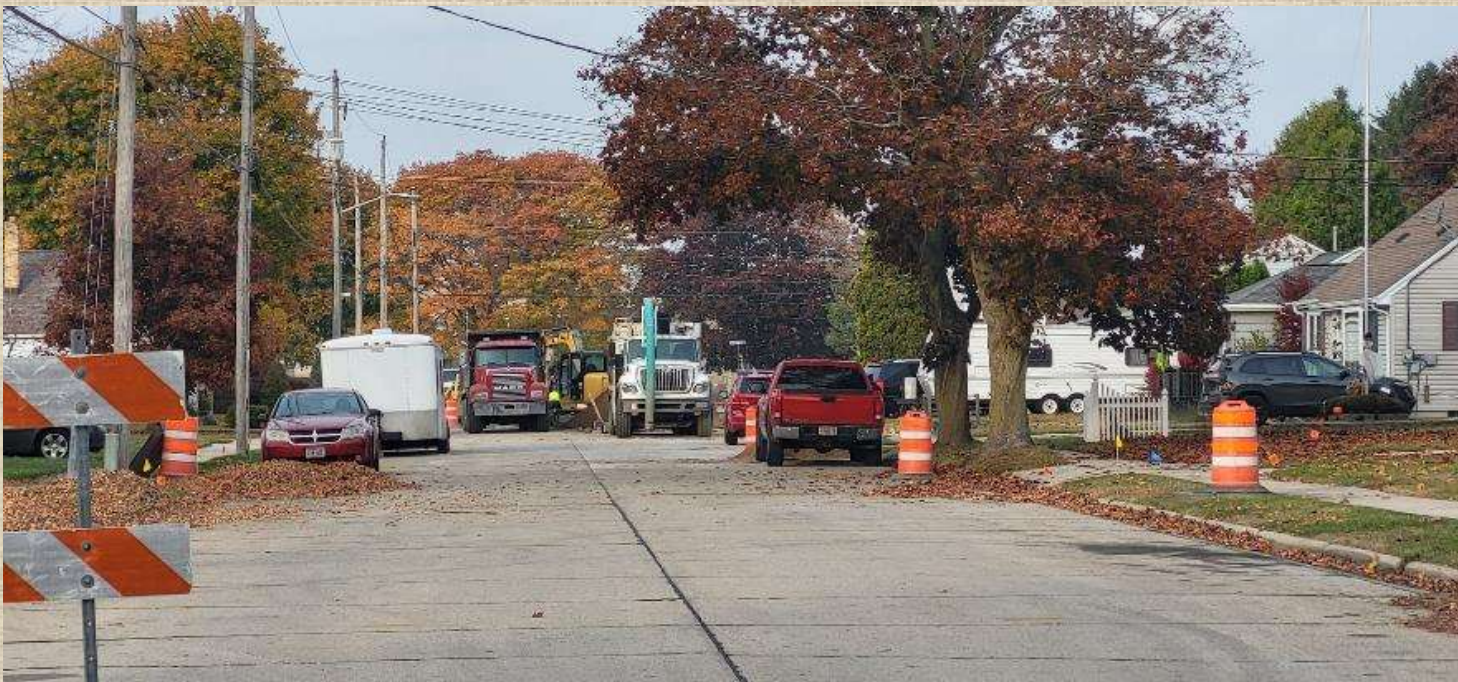
Work is well underway on in the north central area of the City, on 32 nd , 33 rd and 34 th Streets between Tannery Road and Adams Street
